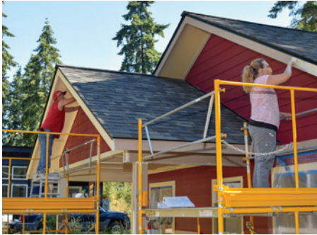
ABOVE: OlyCAP job training participant Jerimah and AmeriCorps service member Echo paint the exterior of a Port Hadlock home. This house, completed in the fall of 2020, is Habitat's 51st in the county.
