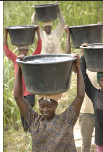
Joyce Asante leads a long line of her fellow villagers carrying water to mix mortar for Habitat homes. Fifty years ago, the old Mowire community in Ghana was dispersed by raiders, and the people have struggled to regain their land and economic viability.
